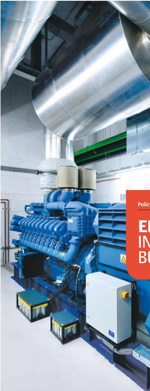
A diesel rotary UPS in the Amstel Business Park data centre, Amsterdam.
